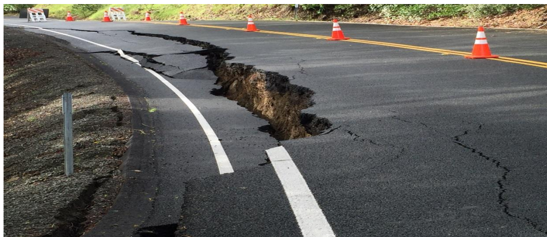
SR-121 roadway in Napa County damaged during weekend storm. (Photo courtesy of Caltrans, March 14, 2006)
